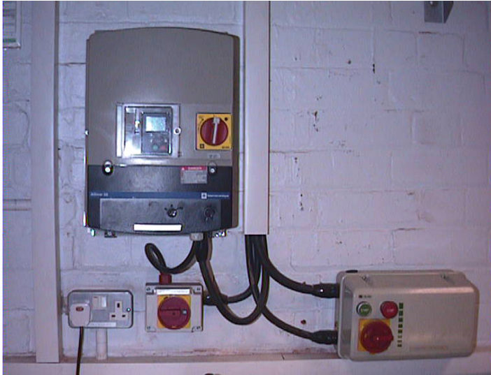
4 KW 3 Phase @ 480Vac Speed Controller
